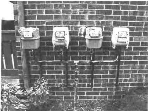
Gas Meters – Located outside Usually on someone's patio
