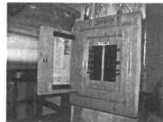
Circuit Breaker Box Inside House
