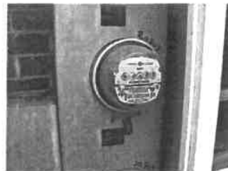
Electric Meter and Main Circuit Breaker
