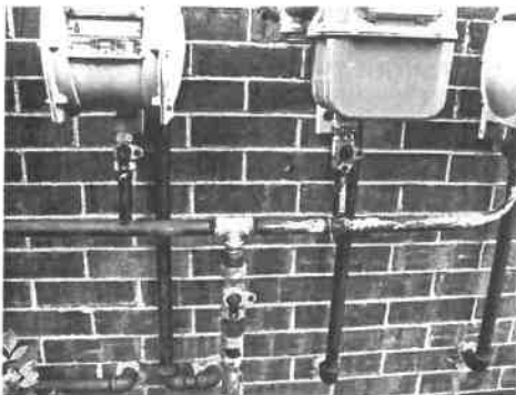
Gas Meter Turn-Off Valve Located under gas meters
