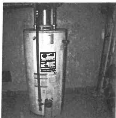
Water Line is Copper Pipe (Upper Right) Gas Line is Black Pipe (Center Left)
